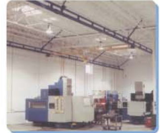
Ceiling Mounted Bridge Cranes & Monorails
