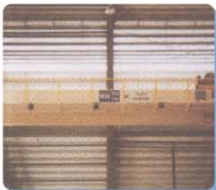
Hoist Crane(Double Girder)
