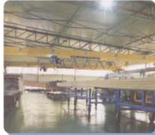
Hoist Crane(Single Girder)
